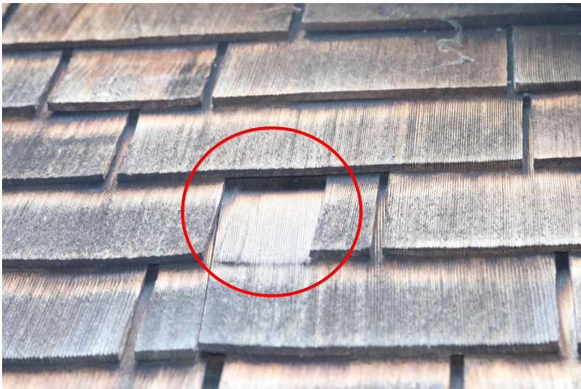
Image 4 – Further missing tiles to the West elevation offering access for bats within
