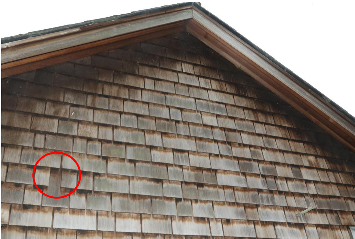
Image 3 – East facing gable elevation of the building offering a single missed tile to the coverings
