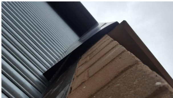
Plate 4.10: Building 2 – Gaps Under Metal Cladding
