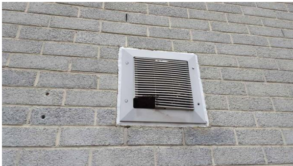
Plate 4.5: Building 1 – Broken Air Vent
