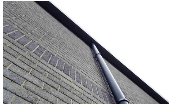
Plate 4.4: Building 1 – Gaps Around Piping
