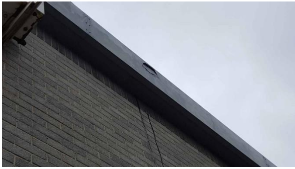
Plate 4.3: Building 1 – Damaged Metal Fascia
