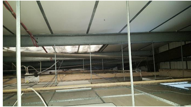
Plate 4.113: Building 2 – Void Above Dropped Ceiling
