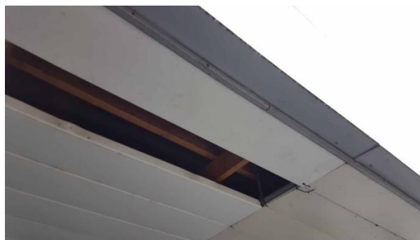
Plate 4.9: Building 2 – Missing Canopy Panel
