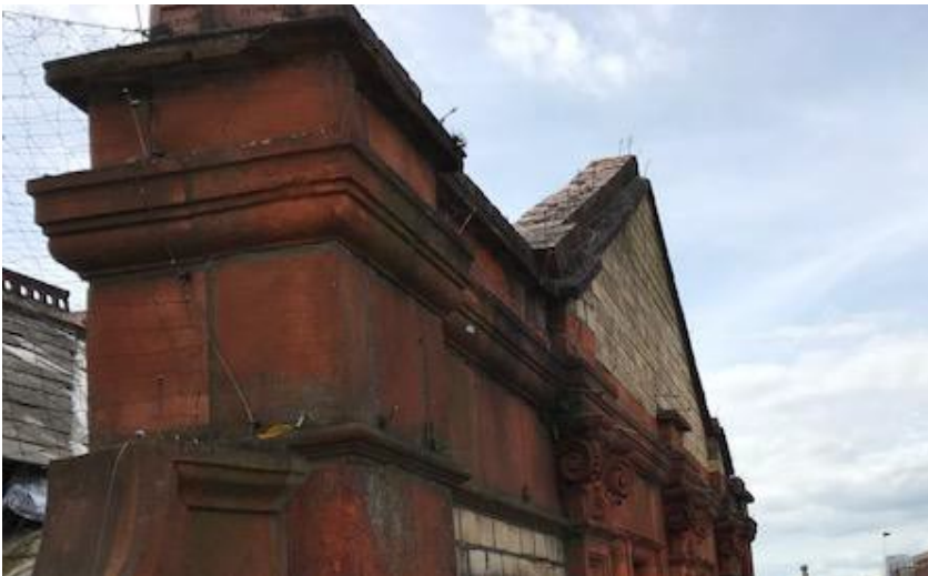
Friars Street Gable with failing brick on edge coping.
