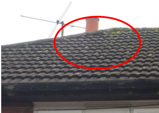
5. Mortar crumbling away from the hip tiles to the rear of the house.
