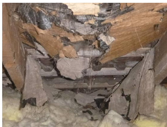
12. The roof with lots of large gaps in the roofing felt.
