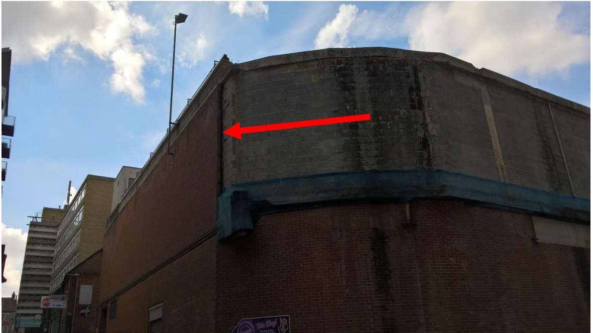
Plate 5 - At the north-eastern corner of B3 a section of brick wall has been removed and this has resulted in the exposure of a cavity wall measuring approximately 10cm wide by 5m high (located denoted by red arrow above). This feature could provide a potential entry point for bats to roost in the cavity wall (TN1) .
