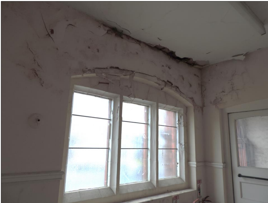
Photo 12 Northeast facing view of damage to vestibule roof caused by damp.
