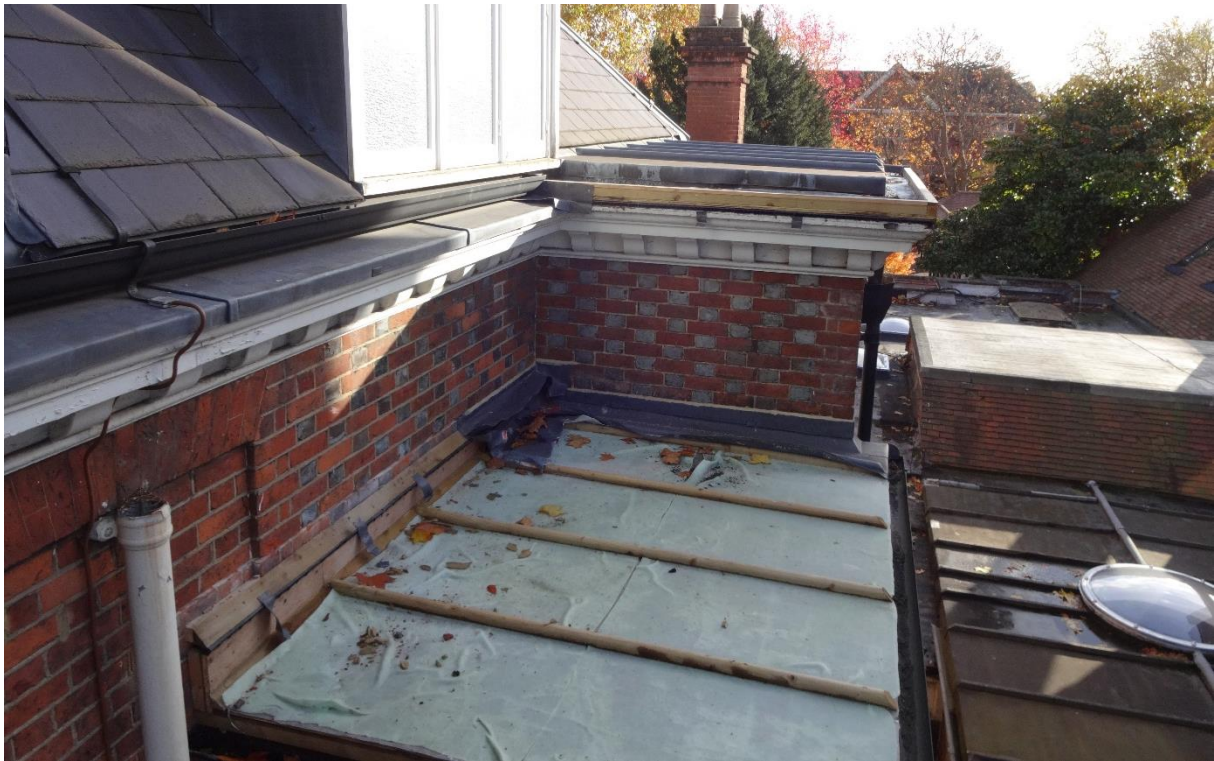
Figure 3: The effected roofs
