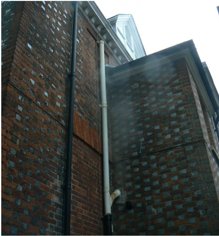
Figure 5: The flat roof in question is on the top of the extension on the right. The soil pipe (white) was probably used to scale on to the roof, but is unnecessarily long
