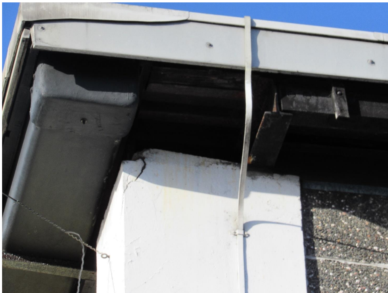
Figure 2. Gap on the exterior of Section 2 of the Central Swimming Pool building, above a concrete pillar and below the guttering. This is the only external feature that was noted on the building.
