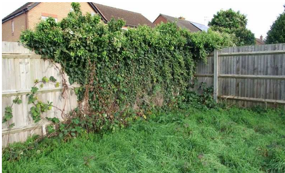
Photograph 8. Small area of ivy growth coming over the northern boundary fence.
