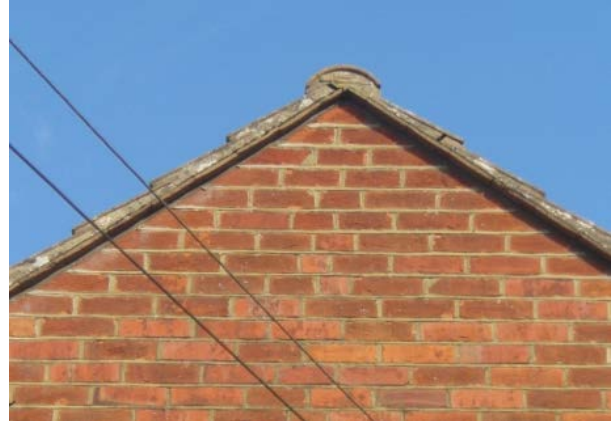
Photo 2: Southern gable apex of Bungalow showing cracks in cement mortar
