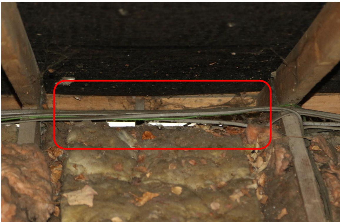
Image 8 – Protruding daylight identified mid-way along the North facing elevation within the eaves
