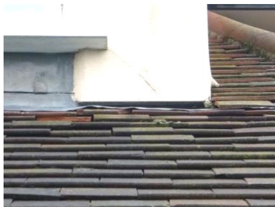
8. Lead flashing lifted by the central window at the front of the house.
