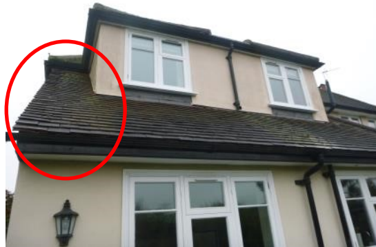
4. Lifted roof tiles towards the verge at the front of the house.
