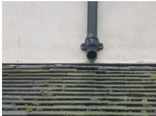
6. Missing roof tile by a pipe at the rear of the house.
