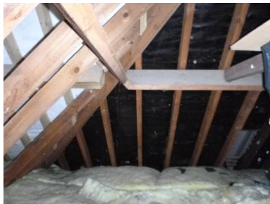
14. The roof space insulated with fibreglass which did not extend as far as the eaves.
