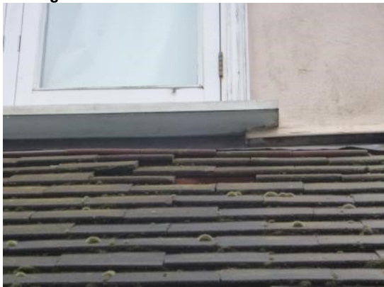
5. Missing and lifted roof tiles below the window at the front of the house.
