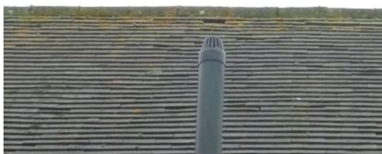
7. Missing roof tile to the rear of the house.
