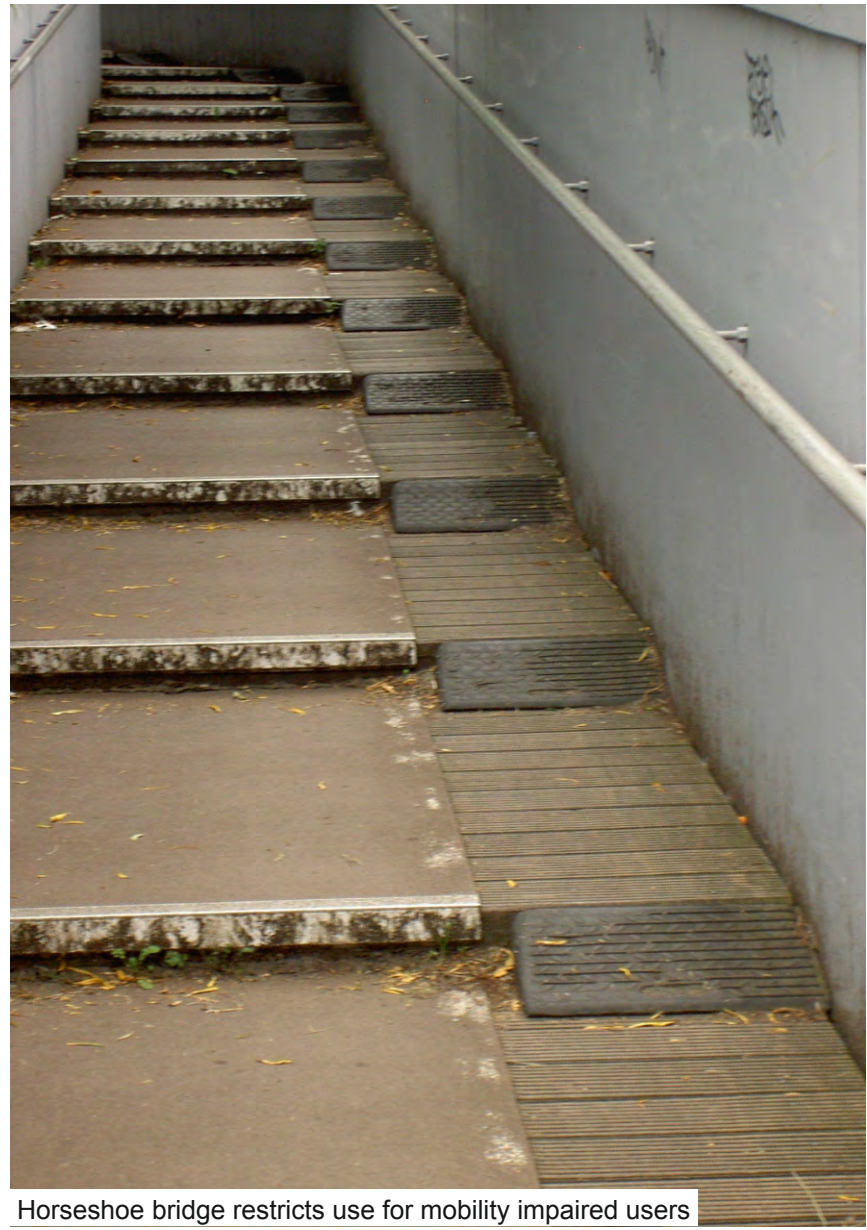
Horseshoe bridge restricts use for mobility impaired users
