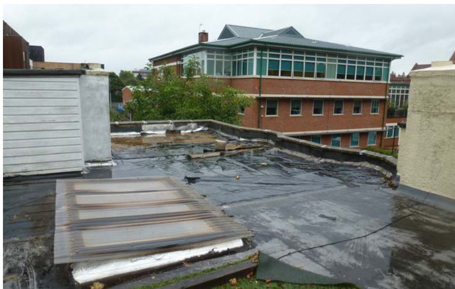
Fig.3: Photograph of existing poor quality flat roof
