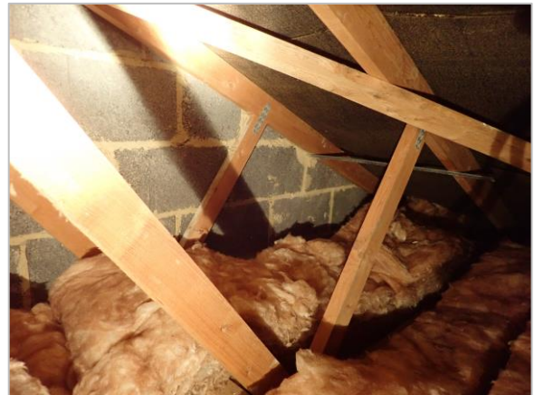
Photo 4 General conditions in loft
