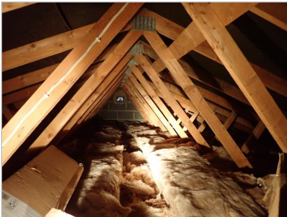
Photo 3 General conditions in loft
