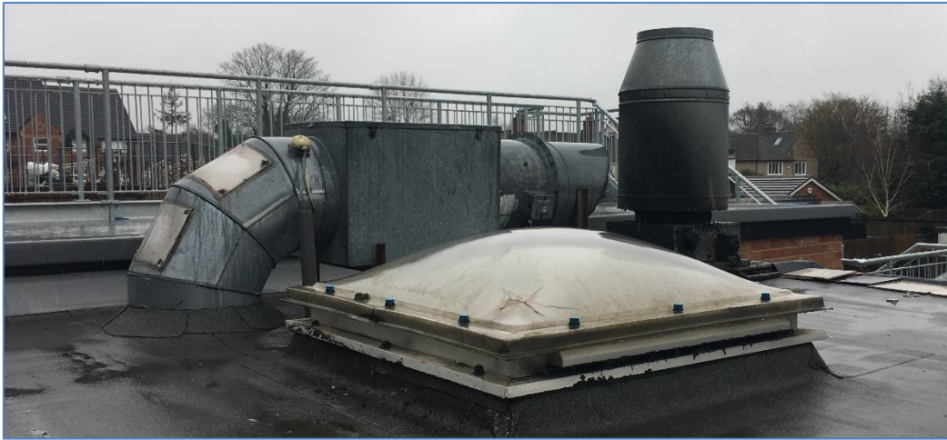
Extract equipment on neighbouring rear flat roof
