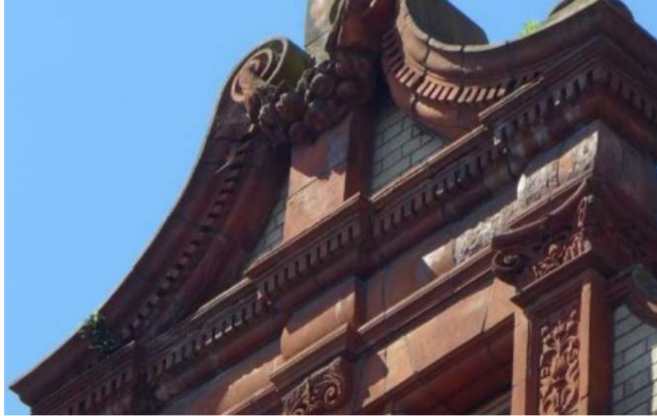
Plate 4.5 Front elevation of Gable at No 21 showing spalling to brickwork
