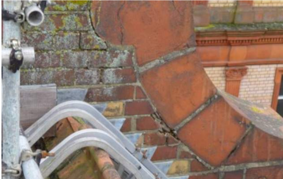
Plate 4.4 Rear of No 15 Gable showing separation of coping from brickwork, mortar deterioration and efflorescence and lichen on bricks
