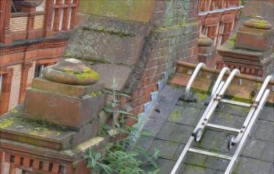
Plate 4.6 Rear of Gable No 17 illustrating presence of vegetation within mortar joints and efflorescence and lichen to brick surfaces
