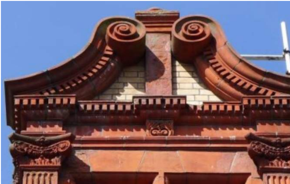
Plate 4.3 Front of Gable at No 17 showing missing elements of corncicing
