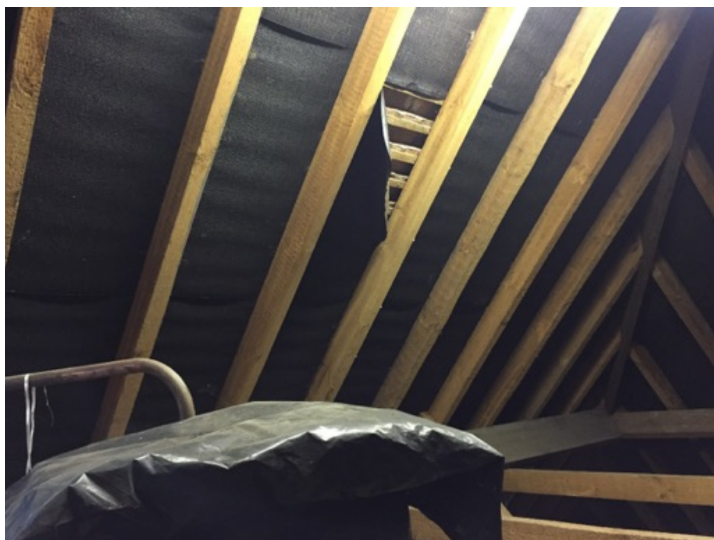
Figure 3. Bitumen lined loft void with occasional tear.
