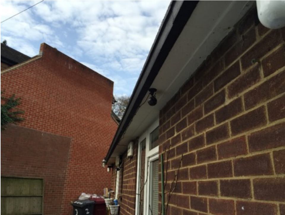
Figure 7. Soffit boards completely sealed.
