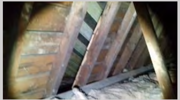
Photograph 10: Building 1 – loft space in Section C facing northeast with missing panel leading into additional void that could not be accessed.
