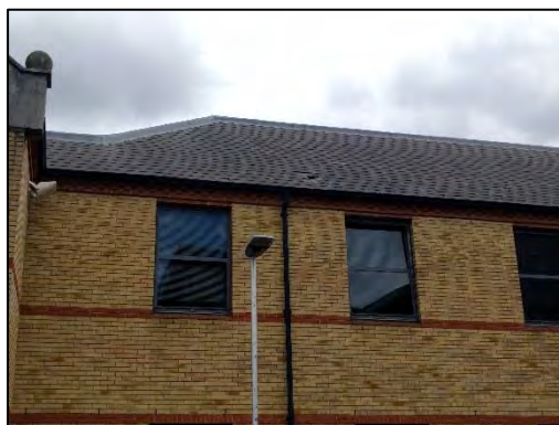
Figure 5: Missing slate tile on western elevation of building
