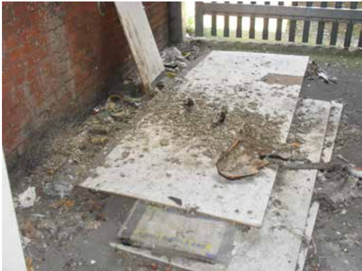
Plate 18: Pigeon guano, pigeon carcasses, wood and other debris within the underpass at Telecom House.
