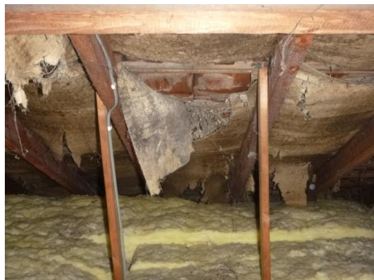
16. Old bitumen roofing felt exposed near the eaves.
