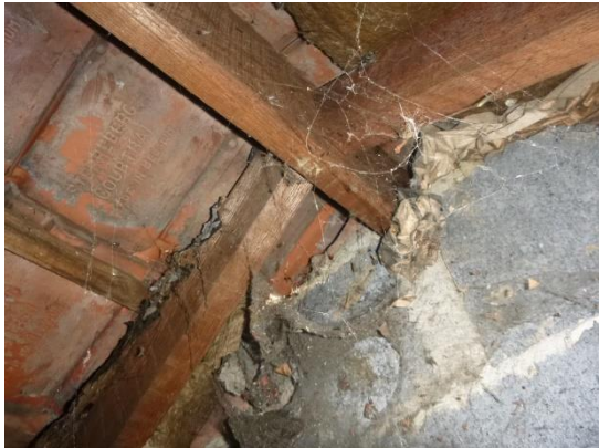
21. Blockwork wall at northwest gable end – cavity insulated with paper but daylight visible through gaps.
