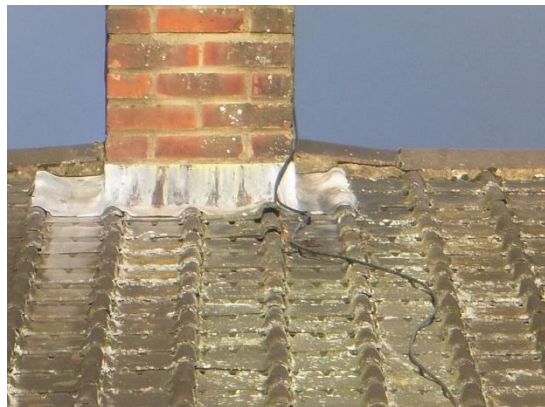
6. Lifted roof tile at the base of the chimney (rear elevation).
