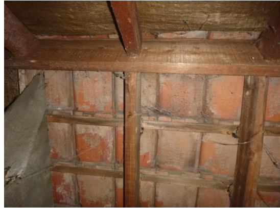
20. Exposed roof tiles west of the chimney.
