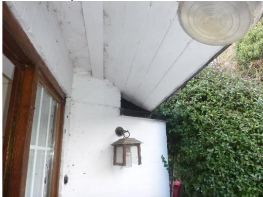
9. Small open cavity between the window and eaves (front elevation).
