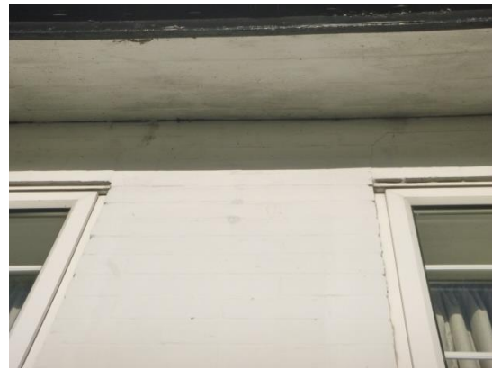
8. Narrow gap behind overhanging eaves (rear elevation).
