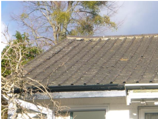
3. Gaps under tiles in proximity to the verge and ridge at the northwestern gable end (rear elevation).
