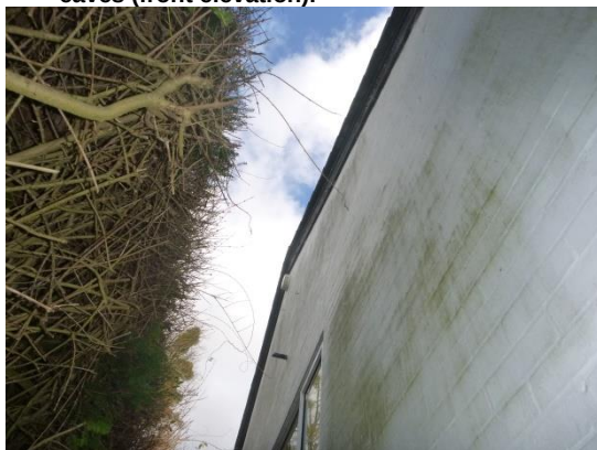
11. Multiple gaps behind barge board on northwestern gable end.
