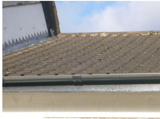
4. Occasional gaps under roof tiles on the southeastern pitched roof (rear elevation).
