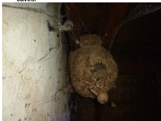
18. Wasps' nest on the western side of the chimney.
