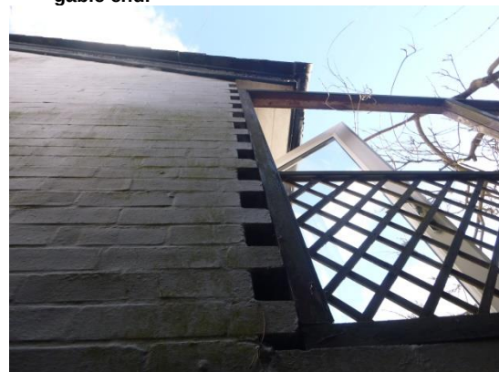
12. Missing bricks on western corner of house.
