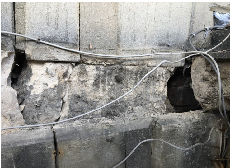
First floor string - face has split off and seems to be supported only on rubble infill, which appears to have settled down. Voids in area obvious.
