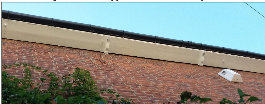
Figure 10 – Image showing boxed eaves, with gap between wall and timber on rear elevation
