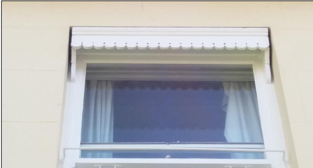
Figure 12 – showing crevices between wall and window lintel on front elevation
