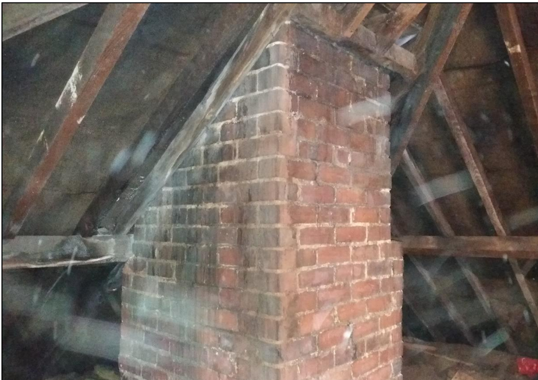
Figure 7 – showing good condition of brickwork on chimney, but signs of staining through damp
