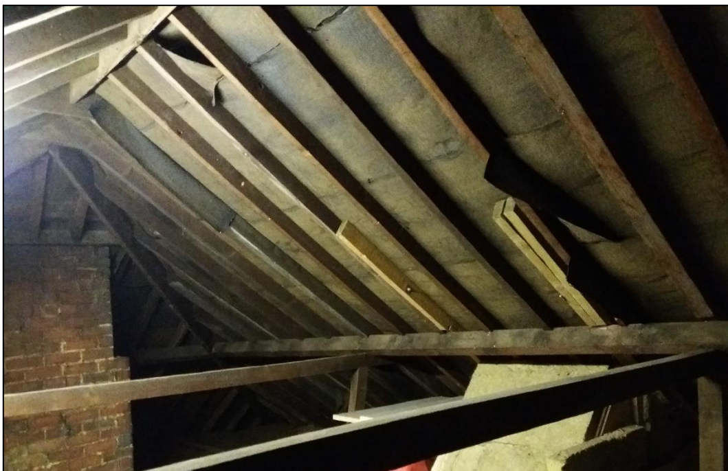
Figure 4 – showing lack of underlay and slates with light entering though gaps (bottom left)
