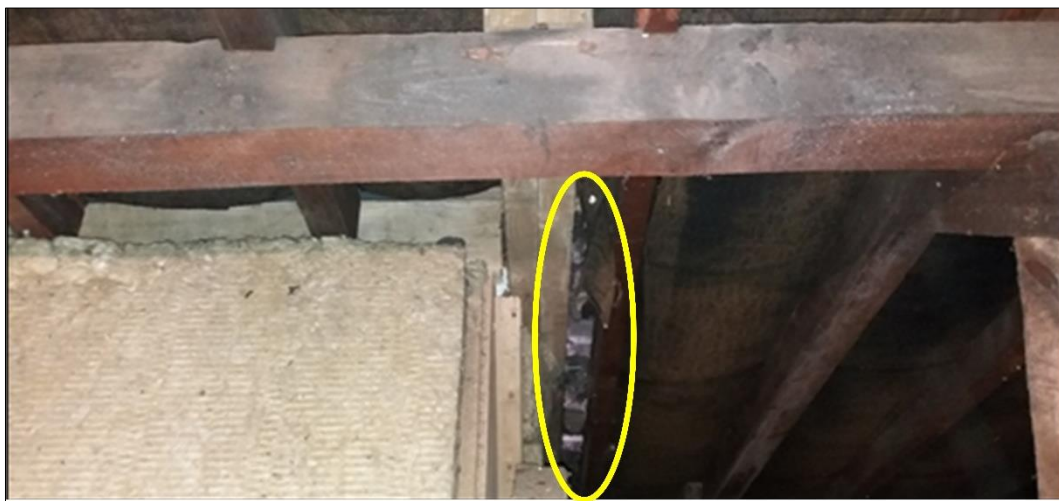
Figure 5 – showing damaged slates, gaps at ridge and signs of damp
