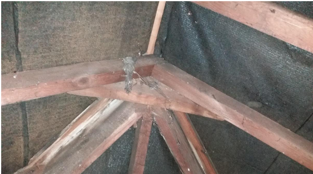
Figure 6 – showing overlaps, dampness and high level of cobwebbing at ridge
