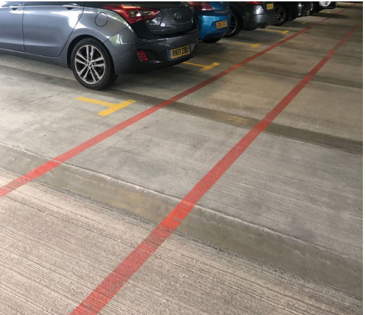
EXISTING CARPARK MARKINGS
