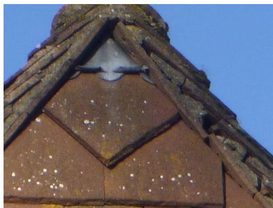
8. Cracks in verge mortar at front gable end (front elevation).
