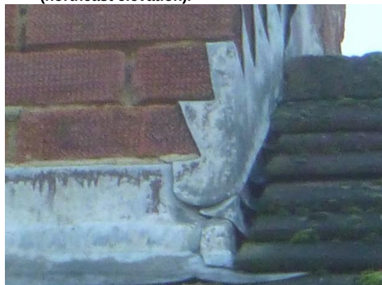
6. Gaps under overlapping lead flashing around chimney (northeast elevation).
