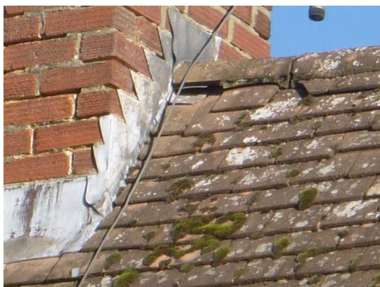
7. Missing roof tile and mortar at ridge next to chimney (southwest elevation).
