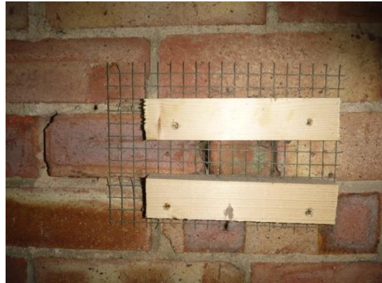
22. Metal mesh and timber over holes in chimney brickwork.
