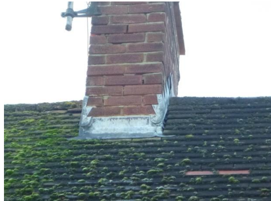
4. Gaps under roof tiles next to chimney (northeast elevation).
