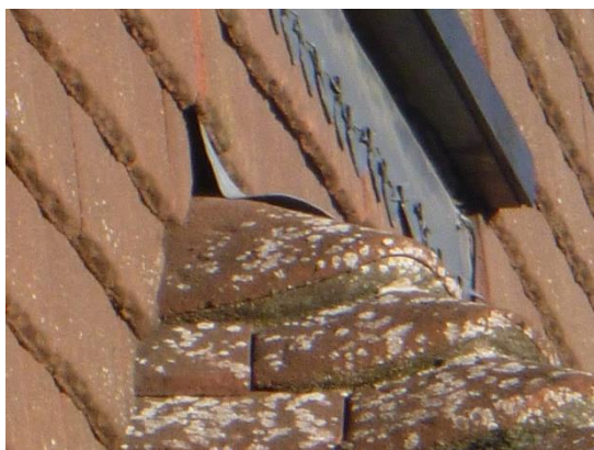
14. Gap under lead flashing lining top of porch roof (front elevation).
