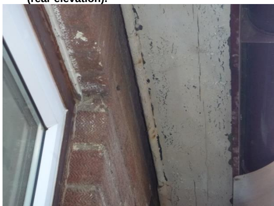
11. Gap between soffit and brickwork (northeast elevation).
