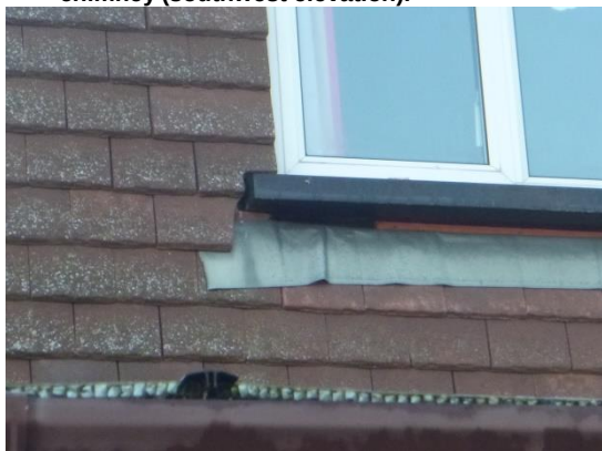
9. Gap behind hanging tiles around window ledge (rear elevation).
