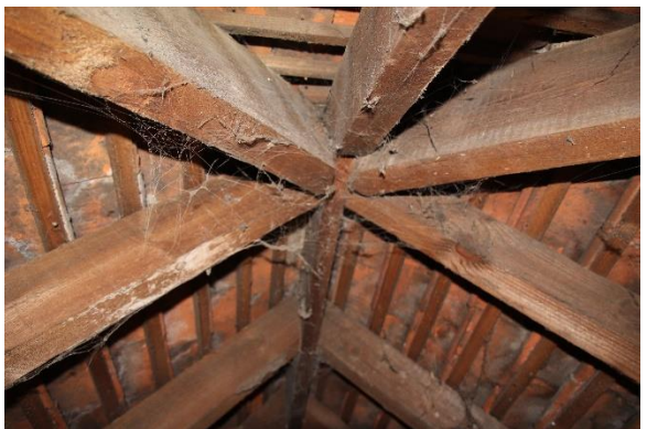
8. Cobwebs at hipped apex
