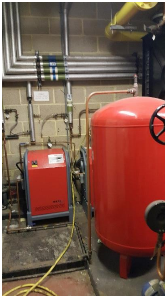
Photograph 9: Gas distribution components in the plant room (second floor)
