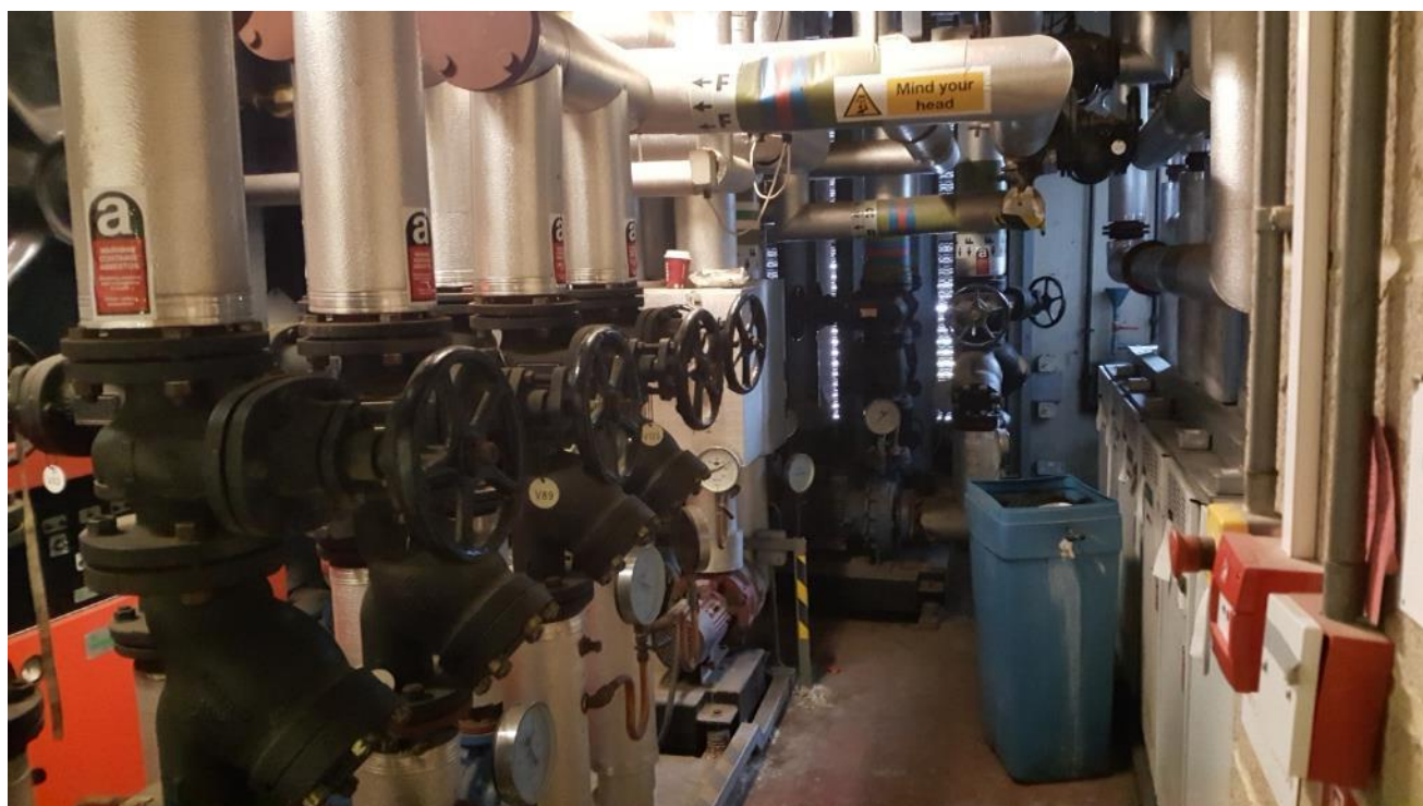
Photograph 10: Gas distribution components in the plant room (second floor)
