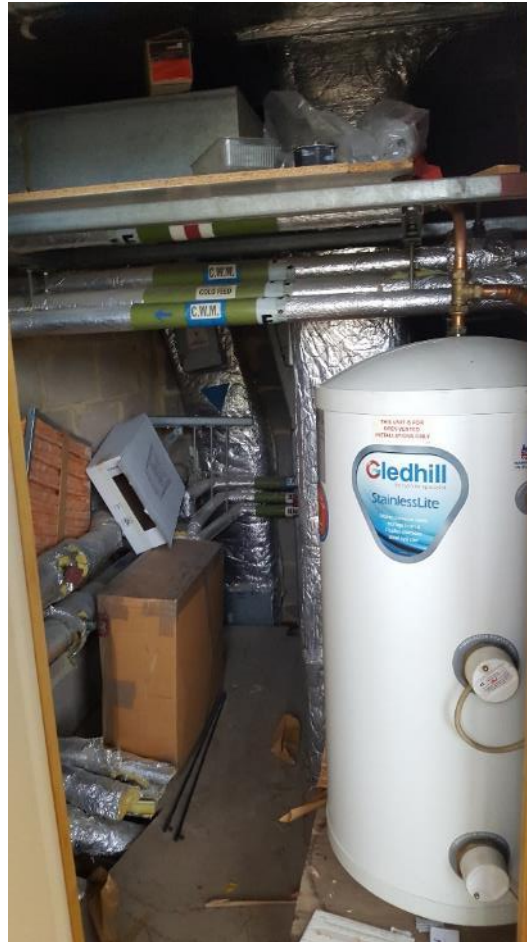
Photograph 7: Plant room within the office building
