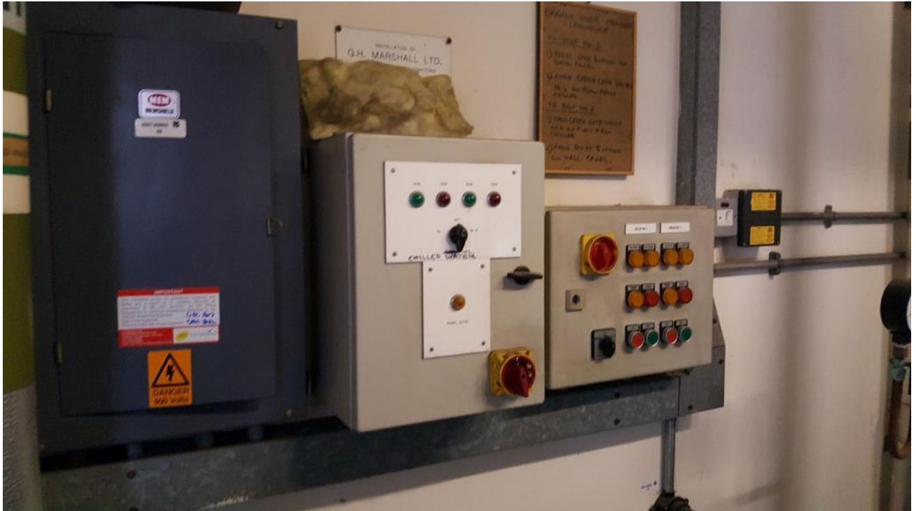
Photograph 11: Electricity distribution components for the chillers (first floor)
