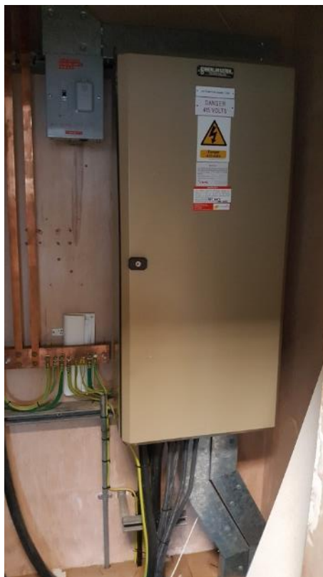
Photograph 13: Typical electrical cabinet
