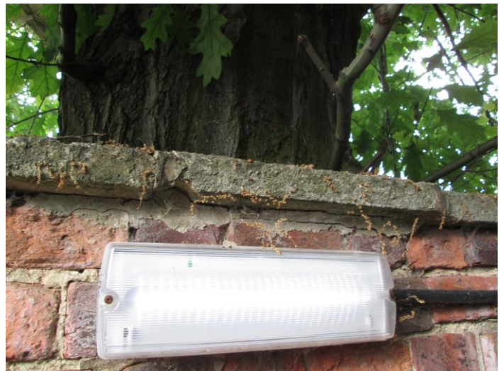
L. T6- touching adjacent brick wall.
