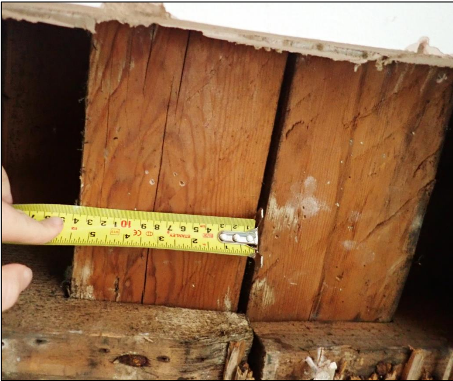
Figure 7. View of the underside of the timber beams which span over the bay window aperture (Note: plaster repairs have been undertaken to the ceiling in this location in the past).
