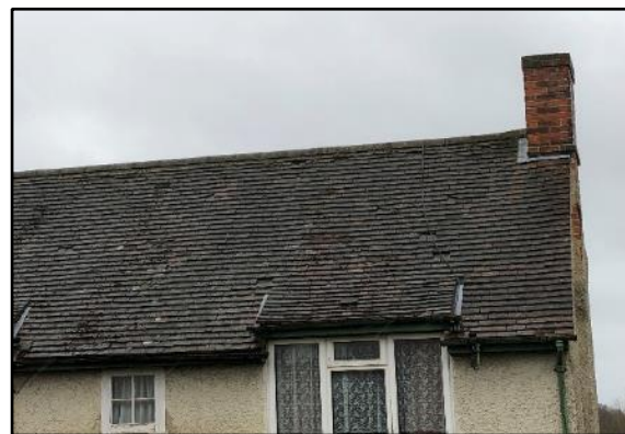
Photo 39: building 203 gaps within tiles on
