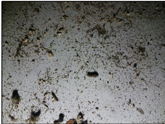
Photo 27:building 199 bat droppings
