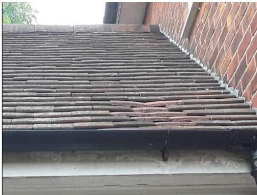
gaps and lifts within rear single storey extension
