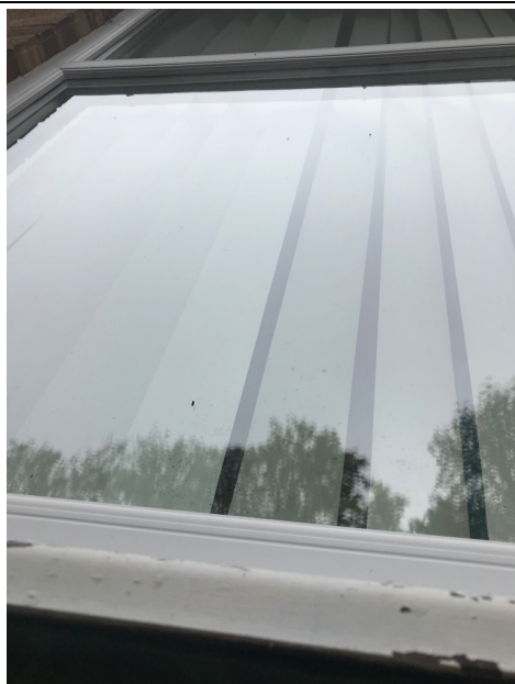
Photo 5 – A few bat droppings on a window on the eastern elevation of No.48
