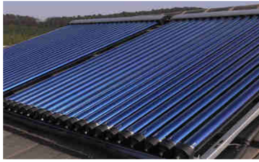
Picture 1: Evacuated tube solar thermal panels
