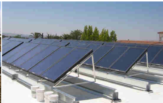
Picture 2: Roof Mounted PV Panels
