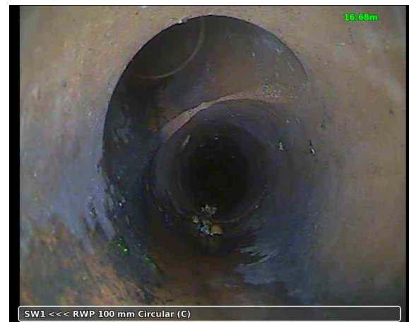
20190529-164610-snap0003.jpg, 00:01:17, 16.68 m Junction, at 09 o'clock, diameter: 100 mm, RWG
