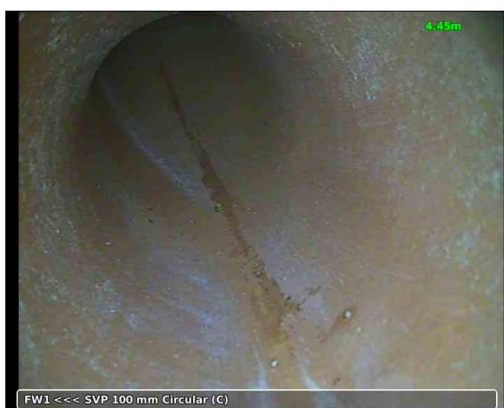
20190529-160922-snap0002.jpg, 00:00:31, 4.45 m Line deviates up
