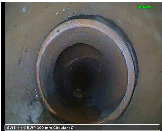
20190529-164610-snap0002.jpg, 00:01:05, 16.61 m Joint displaced, medium
