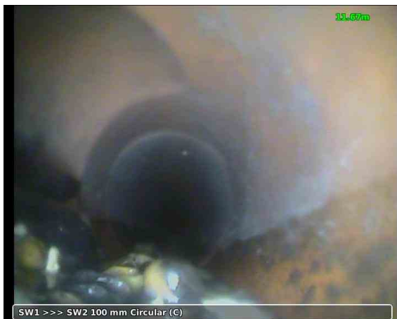
20190529-164119-snap0002.jpg, 00:00:48, 11.67 m Junction, at 09 o'clock, diameter: 100 mm
