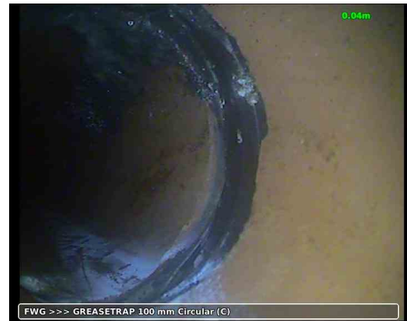
20190529-155231-snap0001.jpg, 00:00:15, 0.04 m Line deviates left
