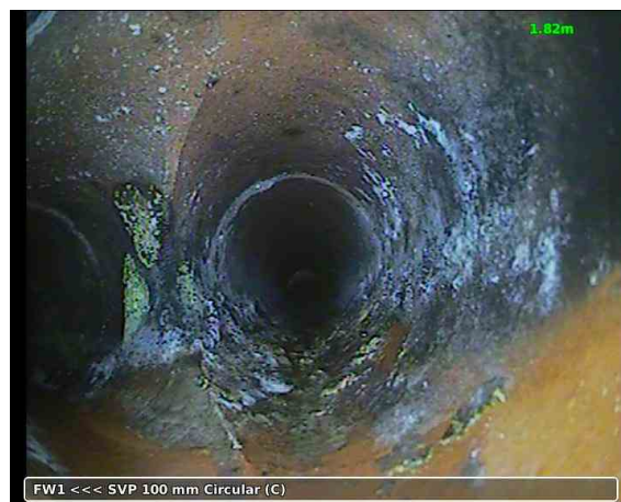
20190529-160922-snap0001.jpg, 00:00:13, 1.82 m Junction, at 09 o'clock, diameter: 100 mm
