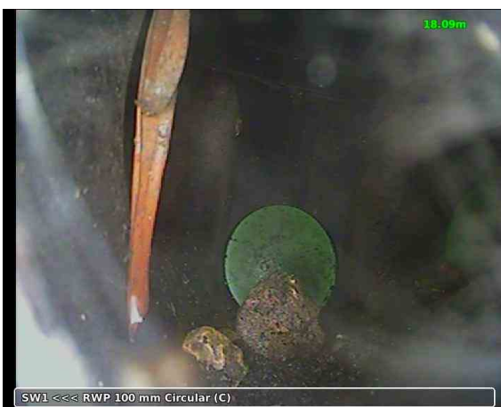
20190529-164610-snap0004.jpg, 00:01:41, 18.05 m Finish node type, manhole, reference number: SW1A, CONCELED CHAMBER
