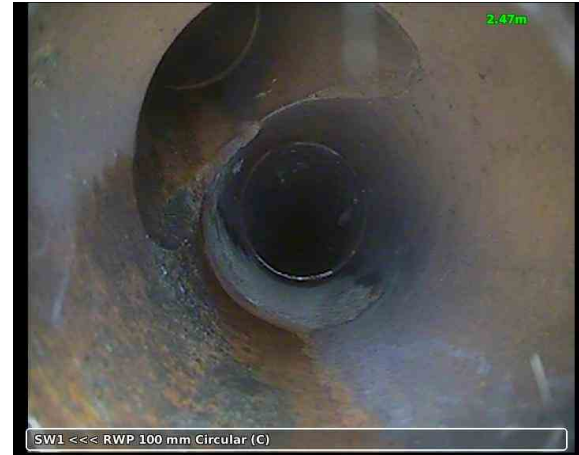
20190529-164610-snap0001.jpg, 00:00:19, 2.47 m Junction, at 09 o'clock, diameter: 100 mm, RWG
