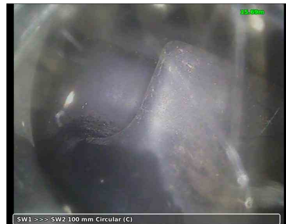
20190529-164119-snap0003.jpg, 00:01:08, 15.69 m Finish node type, manhole, reference number: SW2
