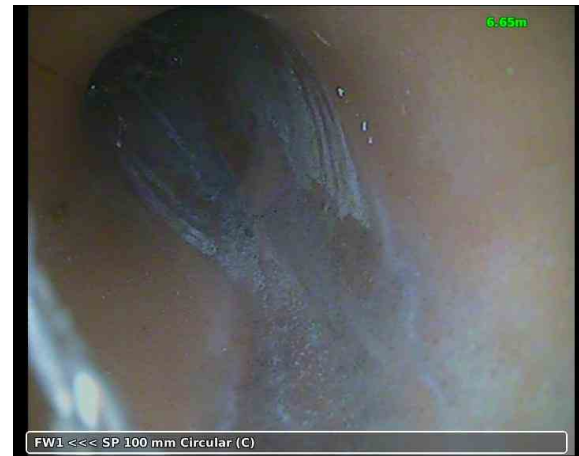
20190529-160652-snap0001.jpg, 00:00:32, 6.65 m Line deviates up
