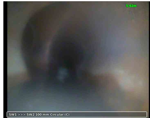
20190529-164119-snap0001.jpg, 00:00:22, 5.59 m Junction, at 09 o'clock, diameter: 100 mm
