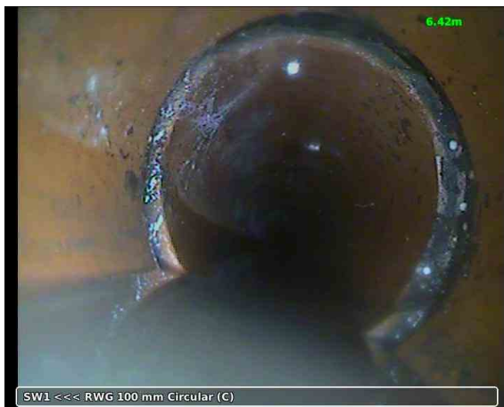
20190529-163553-snap0003.jpg, 00:00:54, 6.42 m Joint displaced, medium
