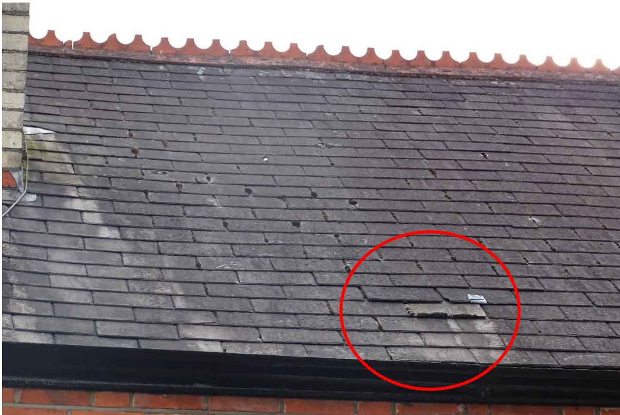
Image 5 – Rear East facing roof coverings demonstrating a lifted area of tiles
