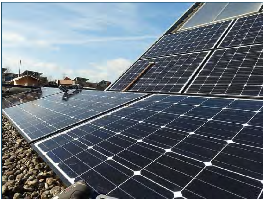
Figure 7.1: PV panels positioned on a south-facing roof space
