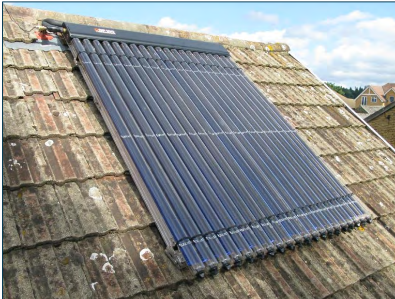
Figure 7.2: A solar water heating panel positioned on the south-facing pitched roof of a house
