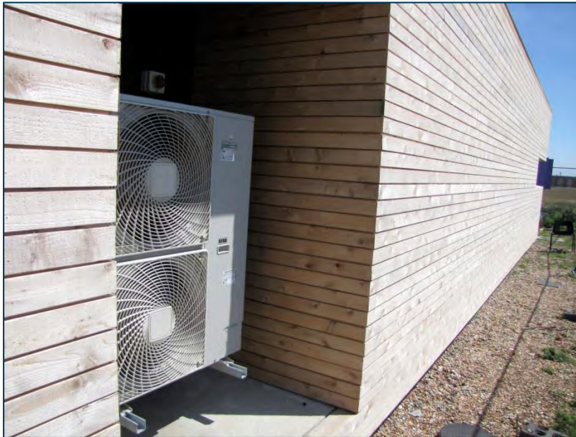
Figure 7.3: Discretely positioned external condensers of an air source heat pump system
