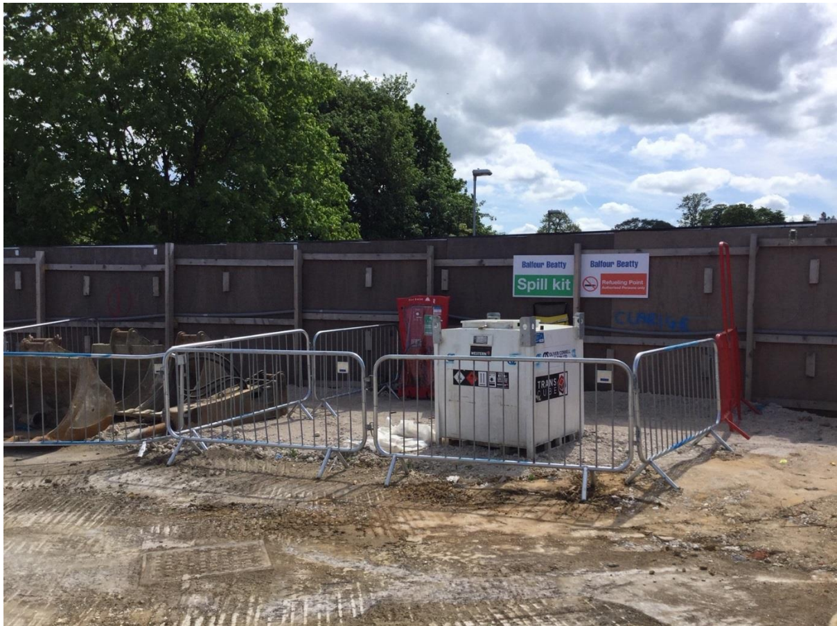
Site re-fuelling area, complete with double bunded fuel tank and spill kit.
