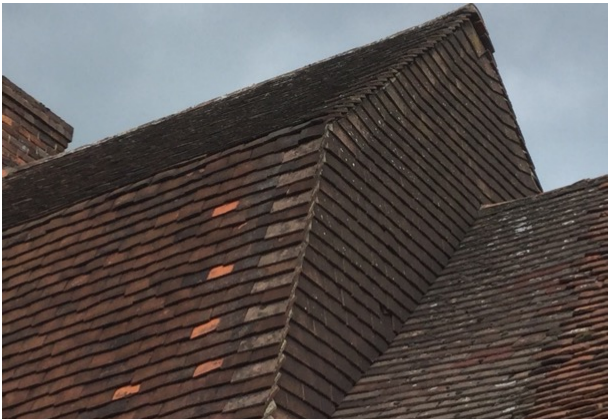
Photograph 4. Areas of looser fitting hanging tiles upon the southern roof gable house at 26-28 Southampton Street.
