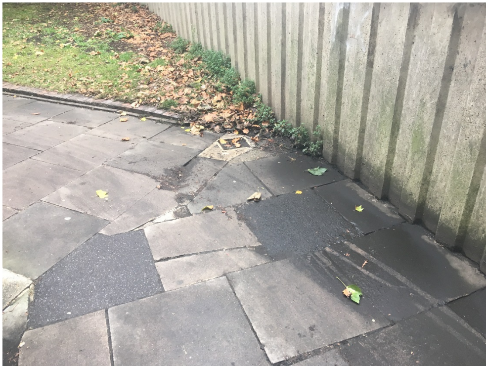
Image 2: Existing footway gully. Clear signs of surface water visible on paving and surface of wall.
