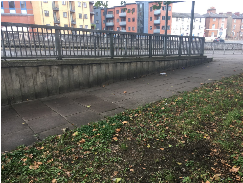
Image 1: View looking North towards A329 from NW corner of Church Hall. Dark lines on wall and paving slabs show signs of past surface water flooding.
