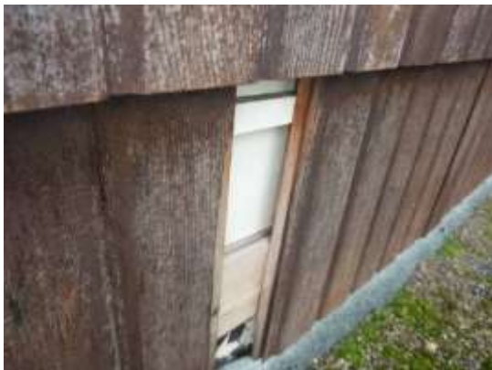
5. Gaps where some of the timber cladding was missing at the western end of the pavilion
