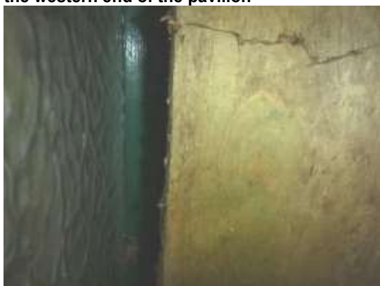
17. Gap between glass and boarding covering the windows to the eastern end of the pavilion
