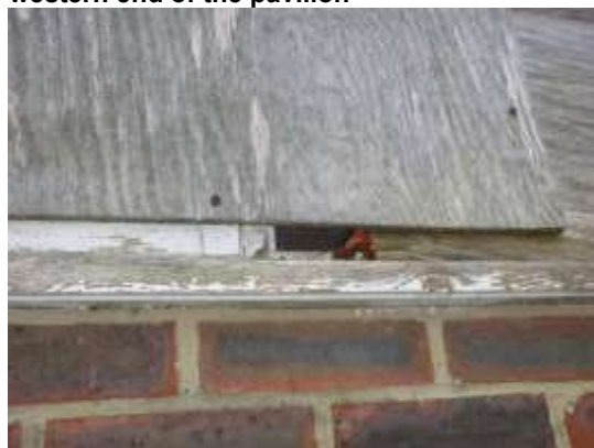
16. Gap behind boarded window to the front of the pavilion
