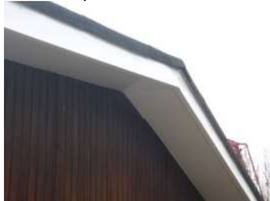
4. Timber cladding tight at the eastern end of the pavilion. Further timber visible behind a gap between the soffit and the cladding.
