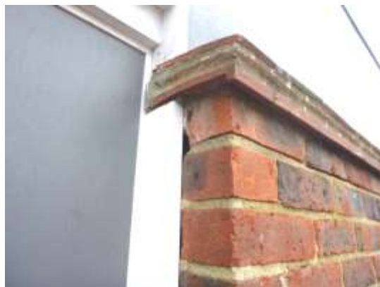
14. Gap behind timber door frame at the western end of the pavilion
