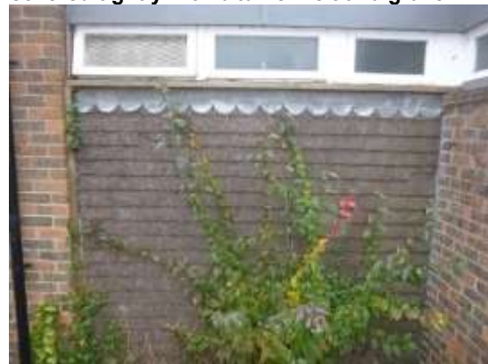
10. Hanging tiles at the western end to the front of the pavilion with vegetation covering some of the tiles
