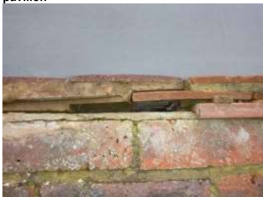
15. Gaps under a small section of roof tiles at the western end of the pavilion
