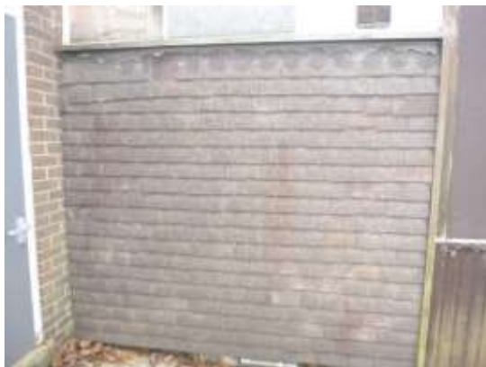
11. Hanging tiles at the eastern end to the front of the pavilion with lead flashing missing and one lifted tile filled with leaves
