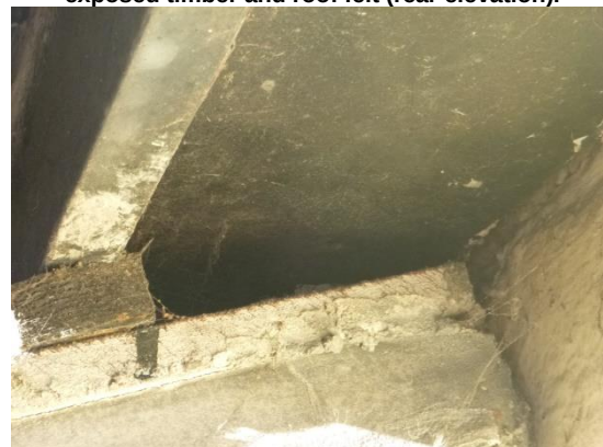
24. Cobwebbed gap behind roof of left-hand window (front elevation).
