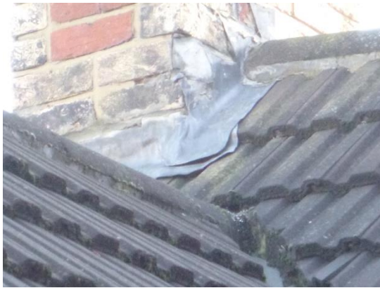
19. Gaps under roof tiles at the top of the roof valley (rear elevation).
