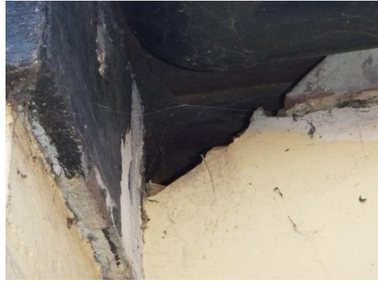
26. Gap in rendered wall (rear elevation).
