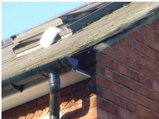
9. End of uPVC soffit box wide open (eastern elevation).
