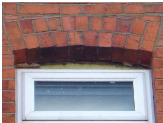
12. Gap behind arched brickwork above right-hand gable end window (eastern elevation).
