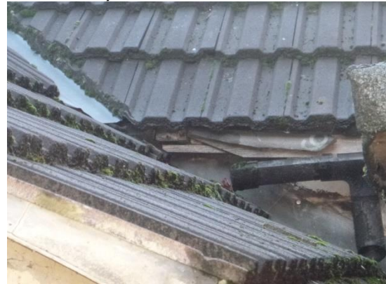
22. Gaps under lead flashing in the roof valley; exposed timber and roof felt (rear elevation).
