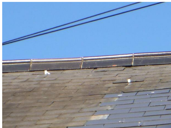
6. Gaps beneath ridge tiles (front elevation).
