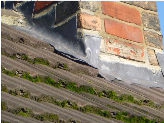
21. Slightly lifted lead flashing around chimney base (front elevation).
