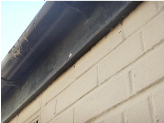
27. Barge board tight to brickwork of eastern flat-roofed extension (rear elevation).
