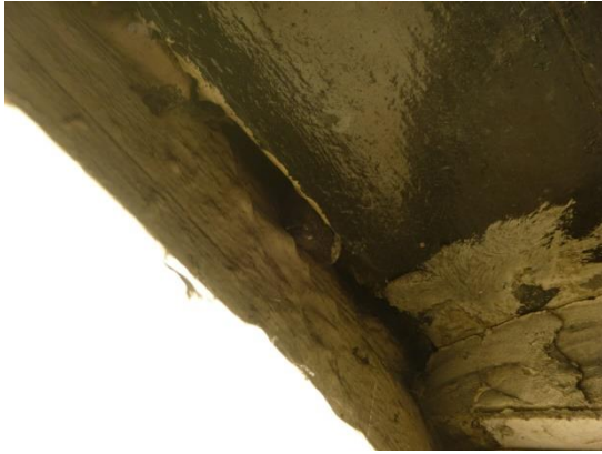
25. Gap behind soffit near left-hand window (front elevation).
