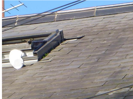
4. Lifted slate tile next to skylight (front elevation).
