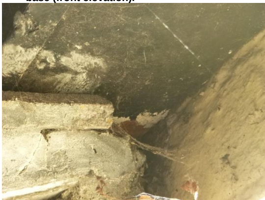
23. Cobwebbed gap behind roof of right-hand window (front elevation).
