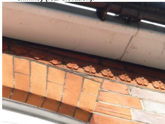
10. Narrow gap behind uPVC soffit (front elevation).
