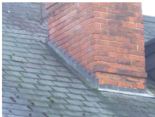
8. Lead flashing slightly lifted at the top corner of chimney (rear elevation).
