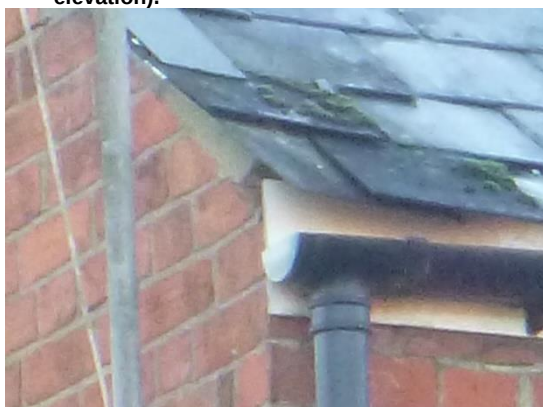
11. Gap at top of barge board at gable end (rear elevation).
