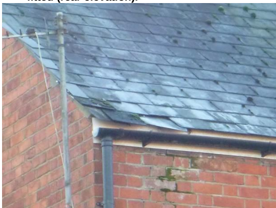
5. Slipped slate tiles (rear elevation).
