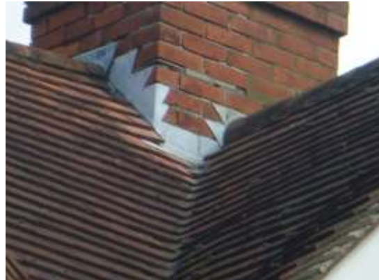
4. Small group of lifted roof tile around the chimney on the front elevation and tight lead flashing.
