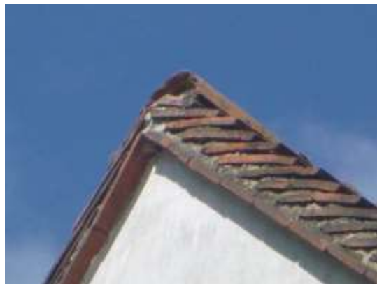
8. Missing mortar at the apex of the rear gable end.
