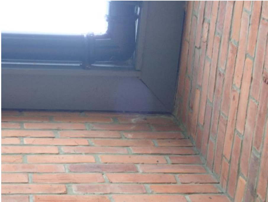
Fig4 gaps between woodwork and brick
