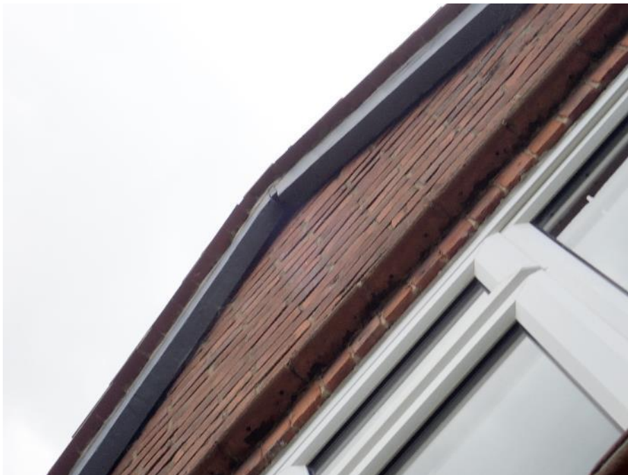
Fig3 – gaps between woodwork and brick
