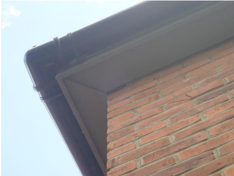
Fig 2 – hole in soffit
