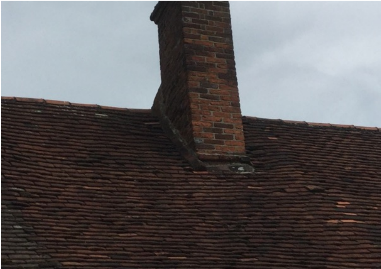
Photograph 5. Areas of loose-fitting roof tiles upon the west facing roof pitch of the building at 26-28 Southampton Street.
