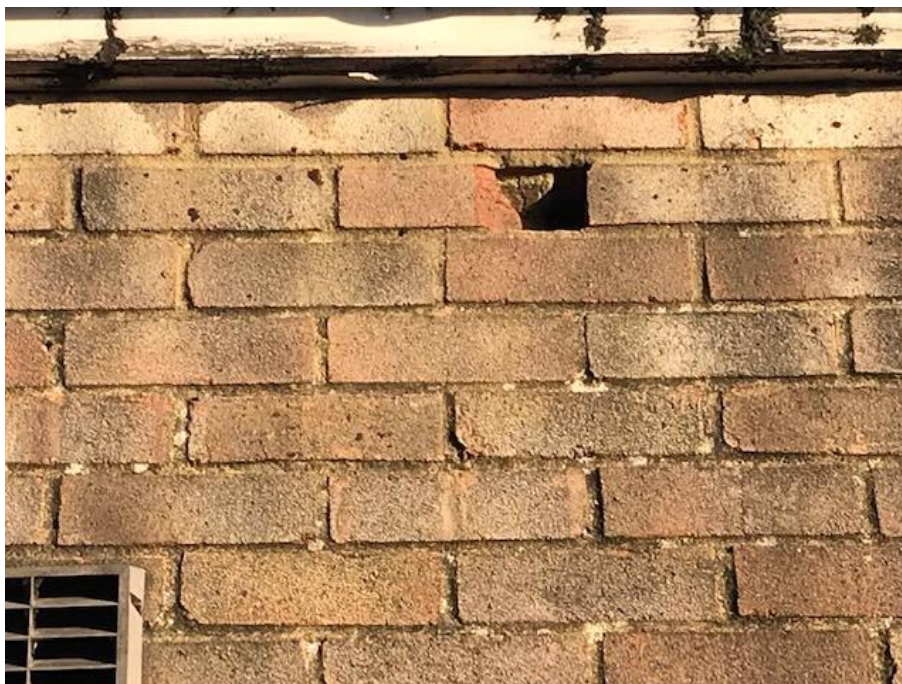
Figure 4.5 Hole in brickwork below fascia possibly leading to internal wall cavity on Building 4.
