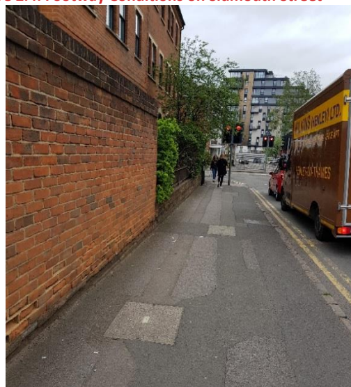
Figure 2.4. Footway Conditions on Sidmouth Street
