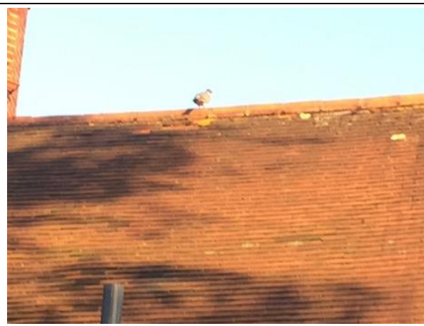
Photo 8: Various gaps under ridge tiles
