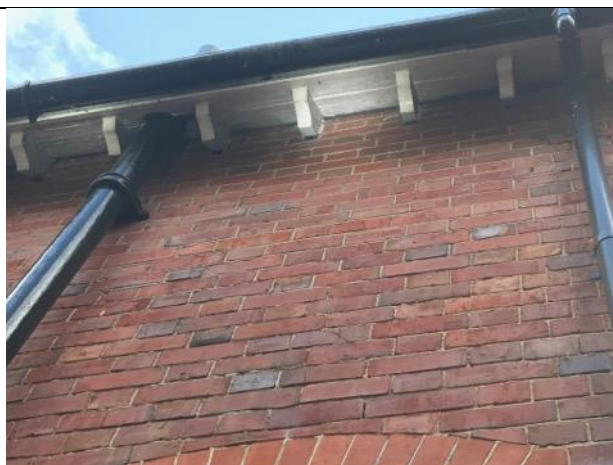
Photo 7: Various gaps under the eaves
