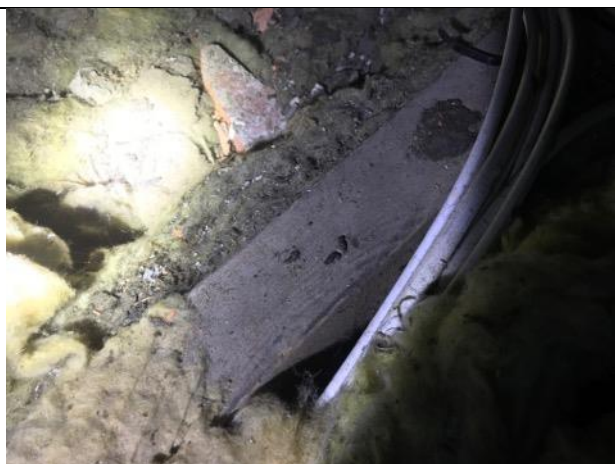
Photo 7: 3 very old bat droppings in loft
