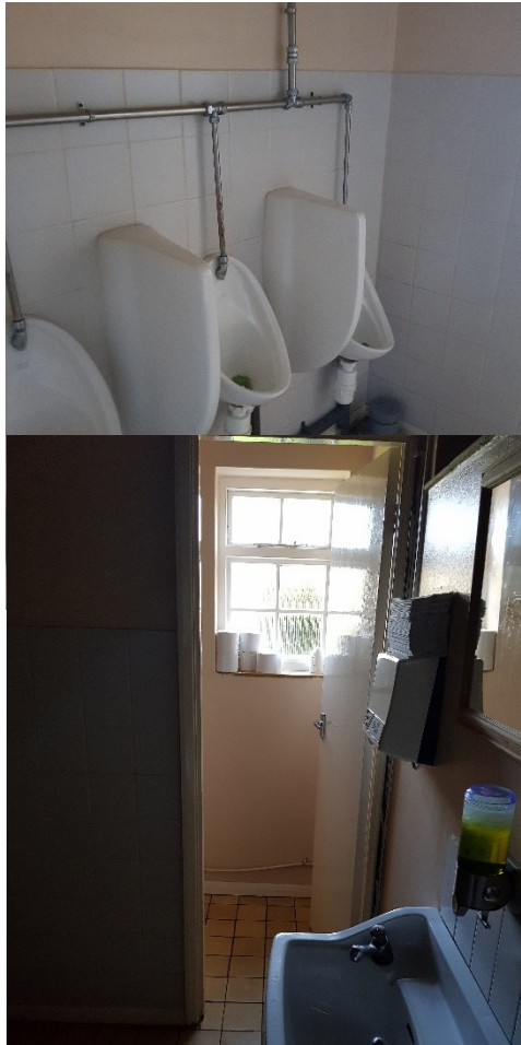
Existing inadequate toilet provision
