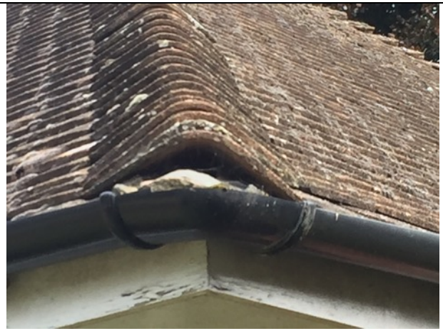
Photo 7 – Missing ridge tile mortar
