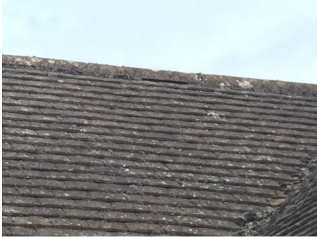
Photo 6 – gap under ridge tile
